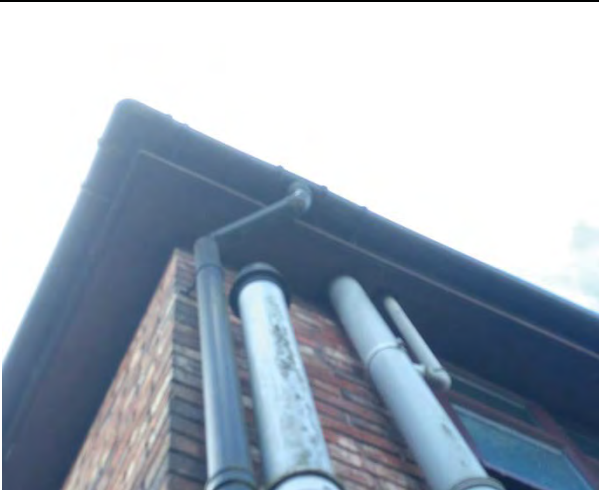
Gap around soil pipe
