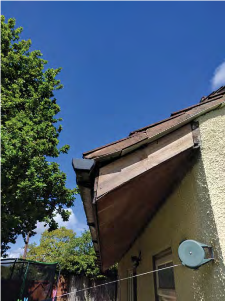
West elevation - Gap between overhanging fascia and undercloak
