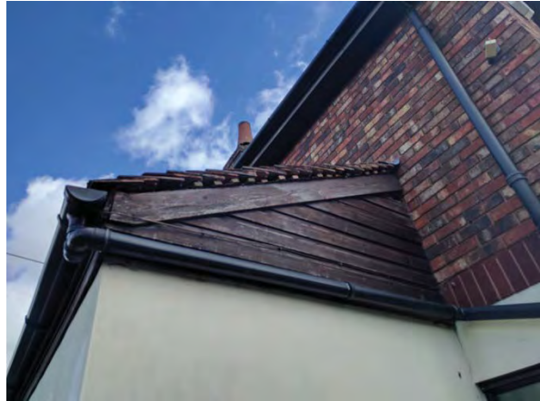
Gaps above fascia board under tiles
