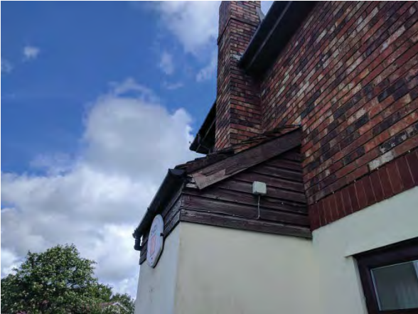
Degraded soffit board and gaps to roof tiles.
