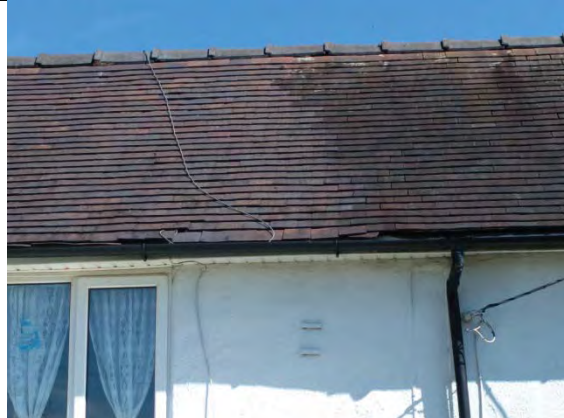
Gaps in ridge tile, slipped tiles by gutter – south elevation.
