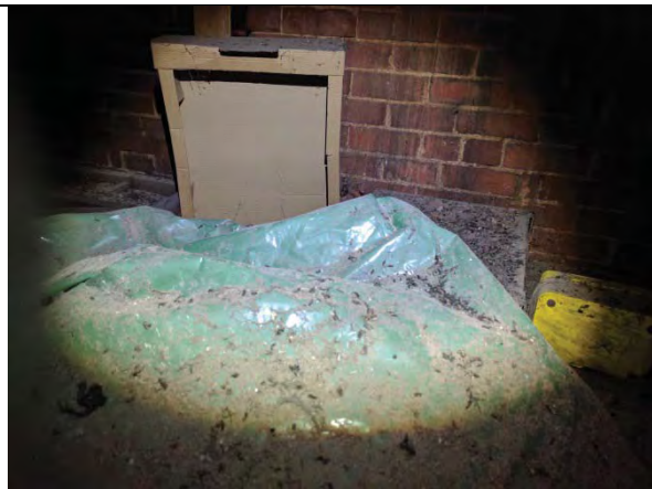
6. Brown long-eared bat droppings concentrated in south west elevation by chimney.
