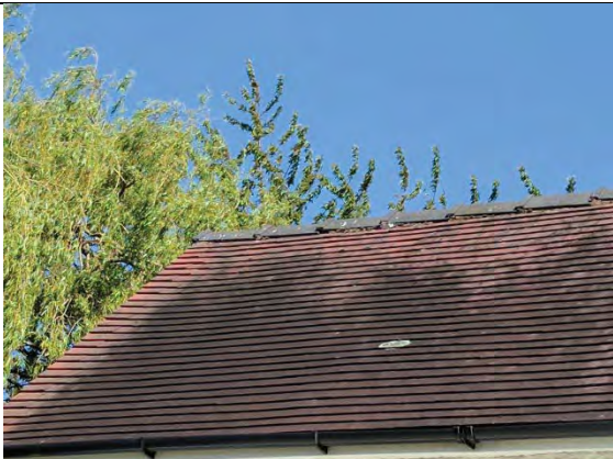
Gaps in ridge tile – south elevation.
