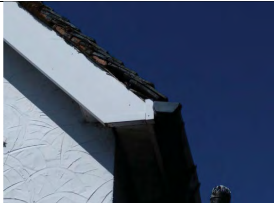
Gaps between roof tile and soffit / fascia. North east and south west elevations.
