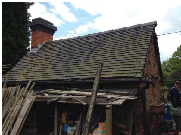
Outbuilding to rear of property. Slipped tiles and gap to ridge tiles. Redundant chimney.
