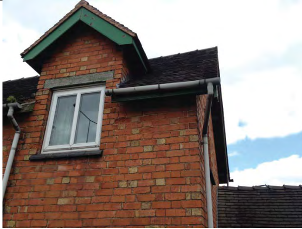
Dormer window to west elevation. Gap above timber lintel.
